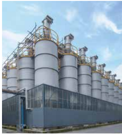
数字化配料系统 Digital Compounding System
