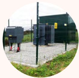
Transformers Increase the voltage.
