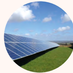
Panels Panels are mounted on steel frames, where steel piles are driven to an approximate depth of 1.5m.
