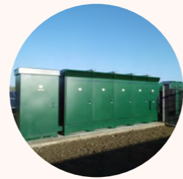
Inverters Convert the Direct Current (DC) into Alternating Current (AC).
