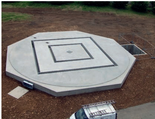
Silo Ventilation ducting shown above prior to silo being built on top hiding this integral feature.
