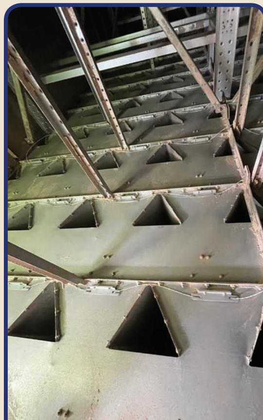
Grain Sentry Fire Detection Cables in position.
