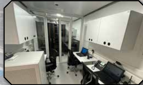
Mobile Communication Unit
