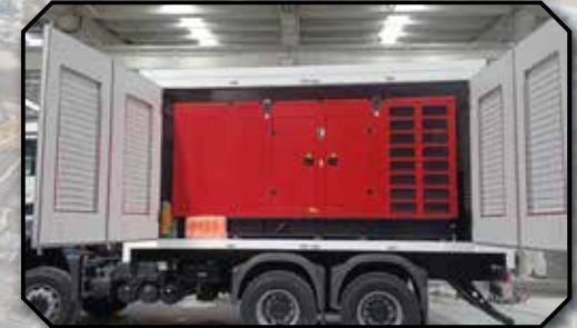
Mobile Generator Unit
