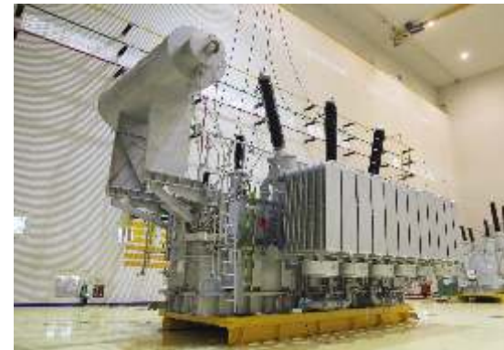
乌兹别克斯坦国家电网公司 新建 220kV zafarabad 数字变电站&扩建 Sirdarya 热电厂两个间隔总包变压器采购 OSFPSZ-250000/220 2台 Uzbekistan State Grid Company: New 220kV zafarabad digital substation built& Expansion of Sirdarya Thermal Power Plant with two spacer general contract transformers purchased OSFPSZ-250000 /220 2 sets
