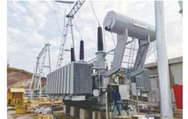
PT.Obsidian Stainless Steel 余热发电工程 2 x 15MW 汽轮发电机组 SF11-20000/35 2 台 PT.Obsidian Stainless Steel Waste heat power generation Project 2 x 15MW steam turbine
