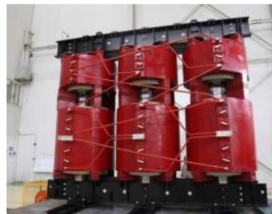
内蒙古东立光伏电子有限公司 年产7500MW太阳能电池组件及配套项目二期年产4.8万吨硅料项目 ZSCB-23000KVA/35KV 33台 Inner Mongolia Dongli Photovoltaic Electronics Co., LTD. Annual output of 7500MW solar cell modules and supporting project Phase II annual output of 48,000 tons of silicon material project ZSCB-23000KVA/35KV 33 sets
