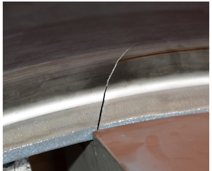
A retaining crack due to torsional vibrations.
