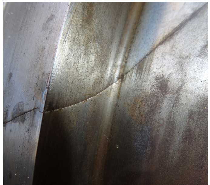
Excessive amplitudes of torsional vibrations can lead to shaft cracking without warning.
