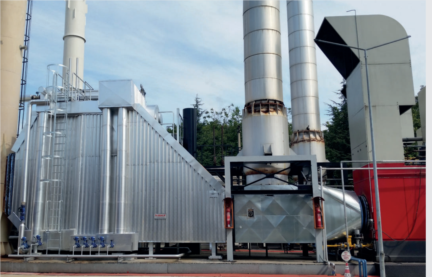
ATIK ISI KAZANI HEAT RECOVERY STEAM GENERATOR (HRSG)
