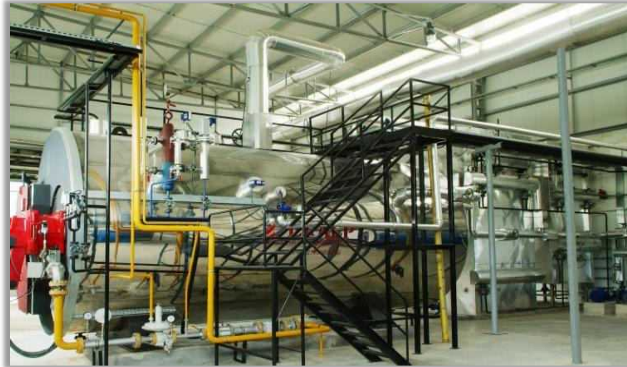
10 ton/h 10 bar Steam Boiler System with 2 economisers
