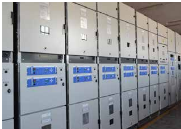
ROMANIA - Cabina primaria bipiano Double tier primary cabin
