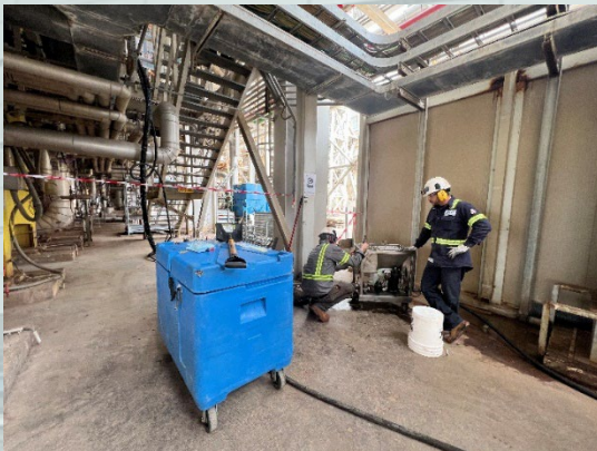
BLASTING MACHINE AND ICE TUBES
