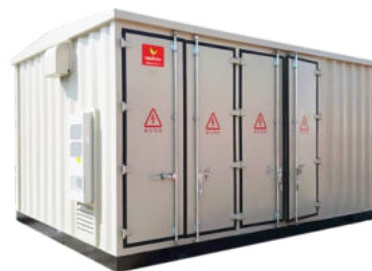
Energy Storage Container
