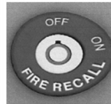
Two-Position Switch (in Remote Location)
