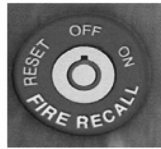
Three-Position Switch (in Elevator Lobby)
