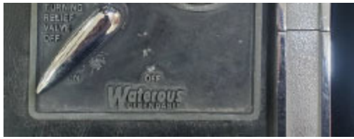
3 A discharge pressure relief valve with indicator lights.
