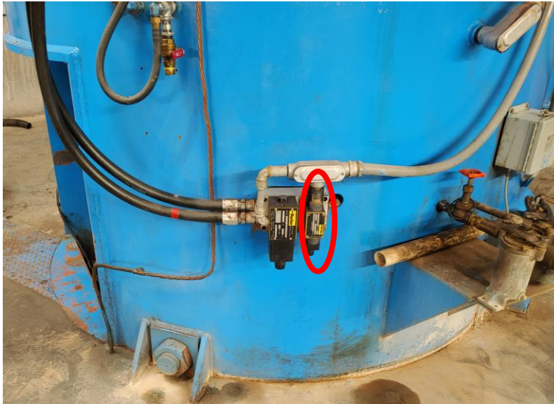
Existing directional control valve
