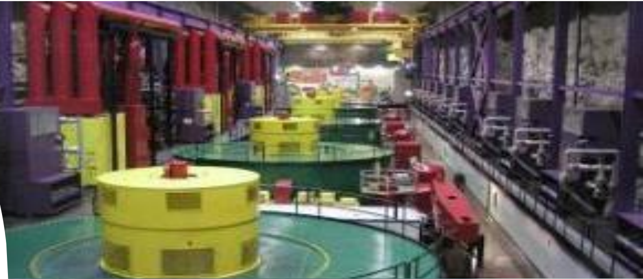
Raccoon Mountain Pumped Storage Project
