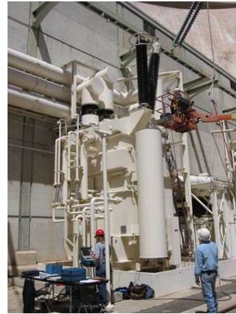
Generator Step Up Transformer
