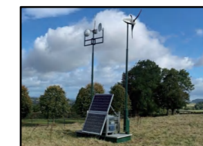
Off grid signal tower
