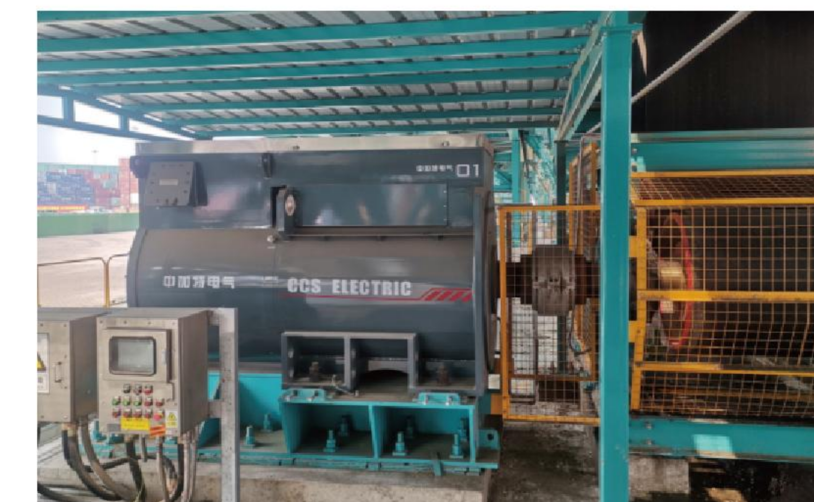
● Grain Belt Conveyor 560kW/10kV Integrated VFD Direct-drive PM Motor
