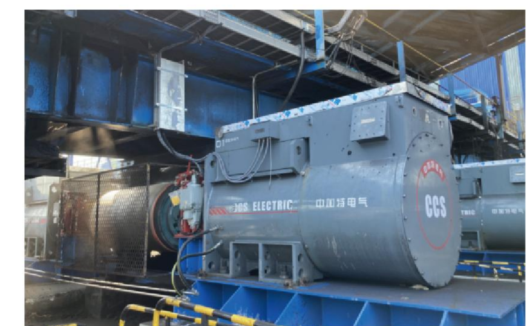
● Coal Belt Conveyor 500kW/6kV Integrated VFD Direct-drive PM Motor
