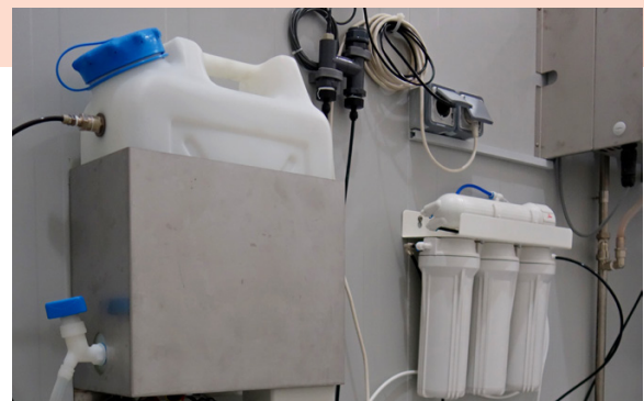
Water Treatment systems
