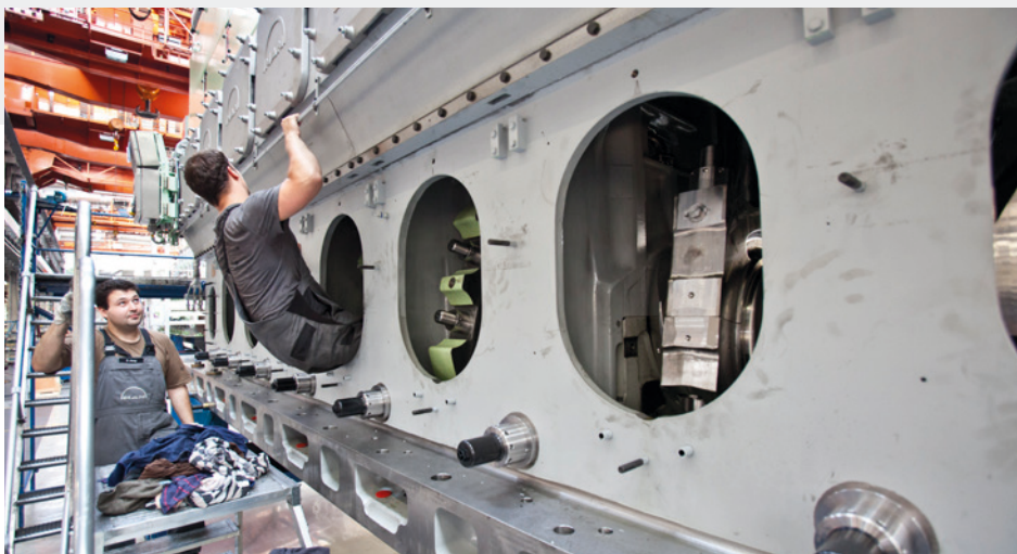
The engines have more than 10,000 hp and are impressive due to their gigantic dimensions.
