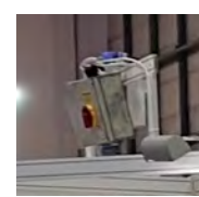
Mains Power Box & Cable Mounted Above Stand
