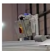
Mains Power Box & Cable Mounted Above Stand
