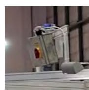
Mains Power Box & Cable Mounted Above Stand
