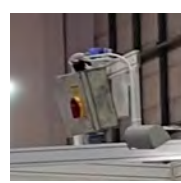
Mains Power Box & Cable Mounted Above Stand
