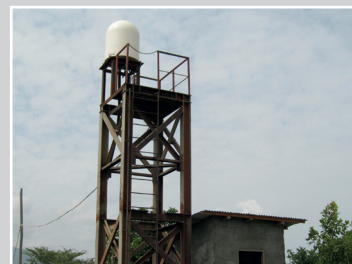
Examples of installations
