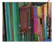
Distressed and weathered colourful cladding
