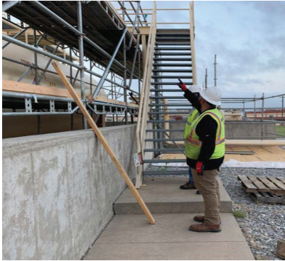
Fig. 6: A coating inspector examined the tanks after work was completed to ensure quality application and curing.
