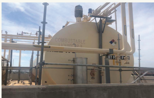
Fig. 1 (top): Seven fuel storage tanks—including these two concrete-encased vessels—required rehabilitation.
