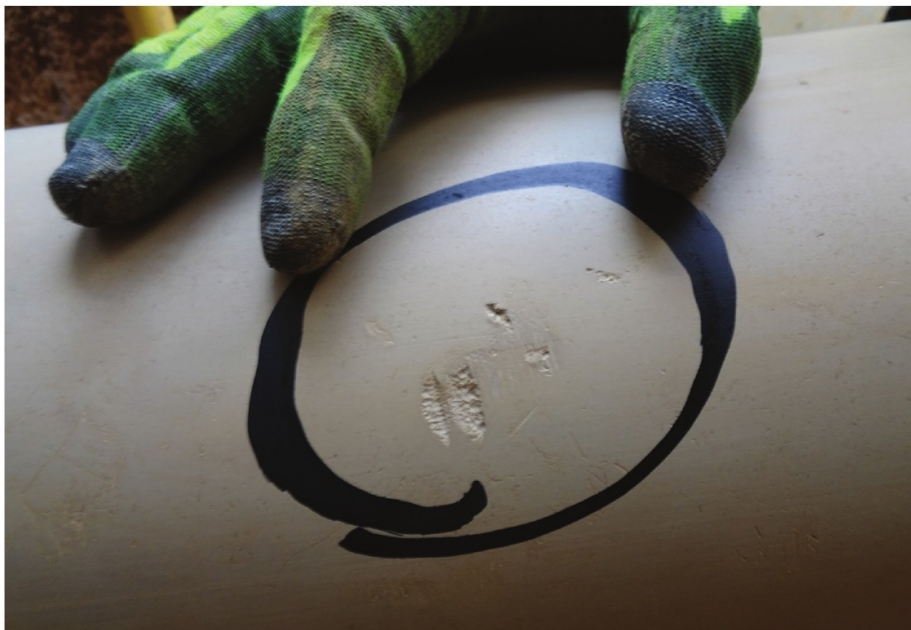
Fig. 4: View of mechanical defect
