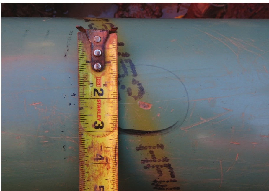
Fig. 5: View of coating defect produced during installation
