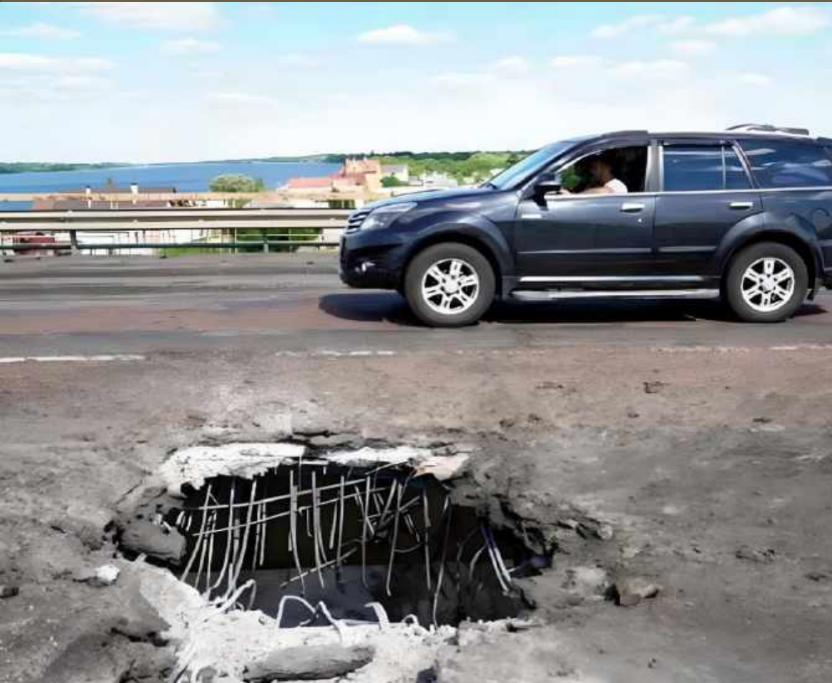
Bridge damage by artillery - Ukraine
