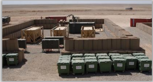
Containerised Power Generation CAT 320 & 350 kVA
