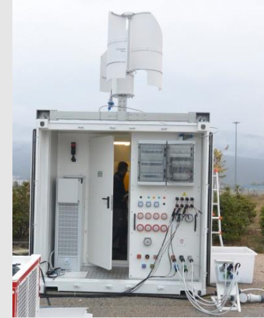
Power Box with wind energy system
