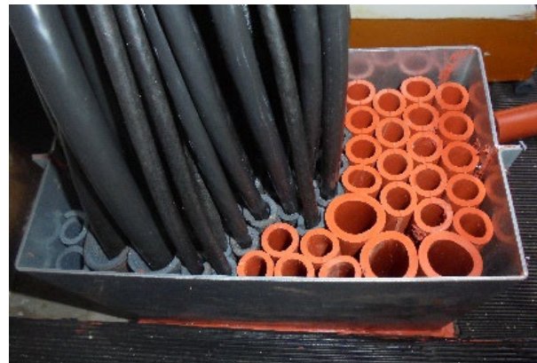
Same 36 cables with RISE NOFIRNO extension frame inserted, space for 26 more cables.
