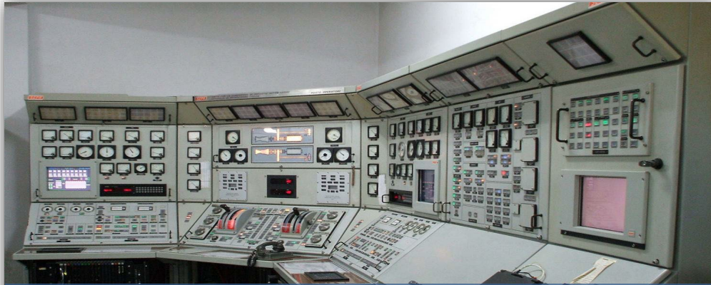
Automation propulsion system
