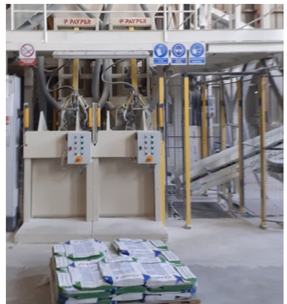
Spillage collector for recycling spilt material
