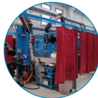
Manual welding stations for certified operators
