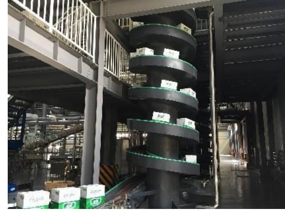
Modular belt spiral conveyor of C'estbon mineral water
