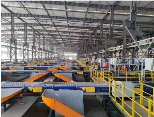
Modular belt conveyor system of China Post in Jinhua East(Zhejiang) Sorting Center
