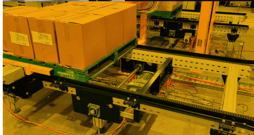
▲ IBC chain conveyor
