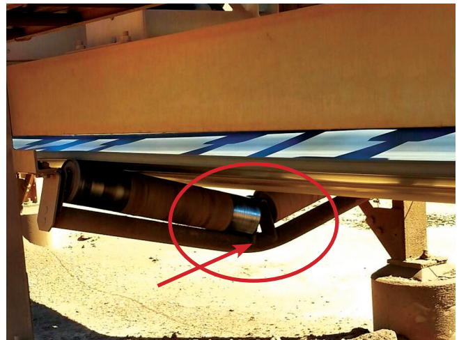
Idler Shell Collapse
