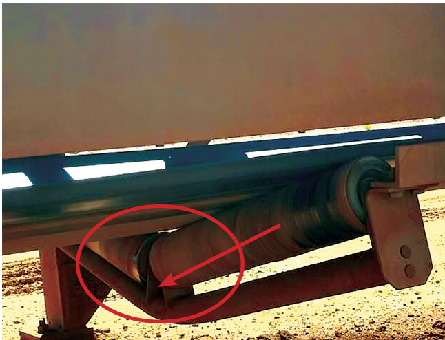
Idler Shell Collapse
