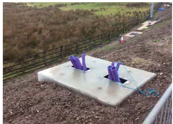
AMI Base on M62 Smart Motorway
