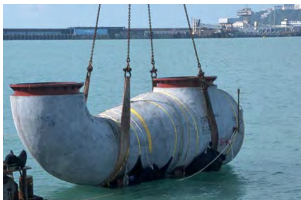
Long Sea Outfall Diffuser
