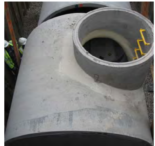
Circular Attenuation Tank with side entry manhole
