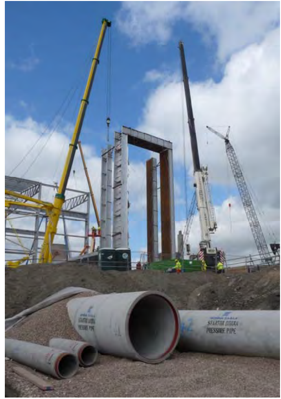
West Burton CCGT Power Station cooling water pipework
