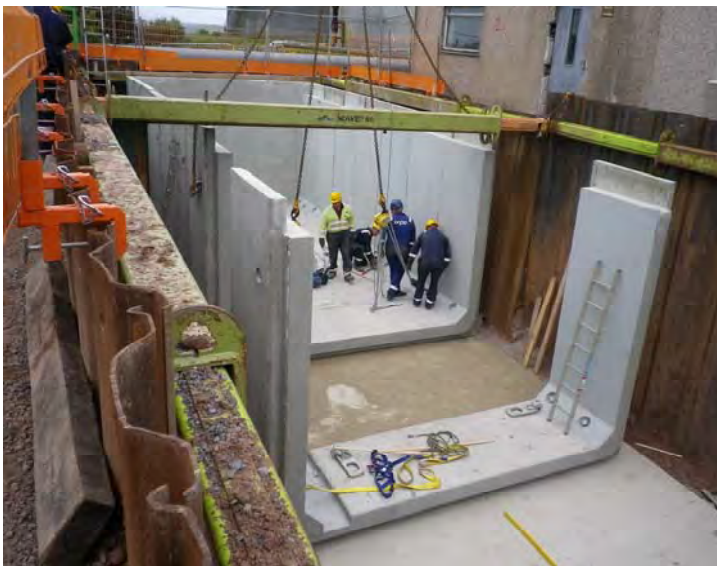
Bespoke trough used at Valero Pembroke Refinery
