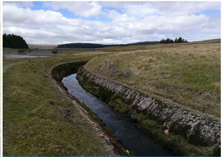
Algae, moss & vegetation growth within the flume channel
