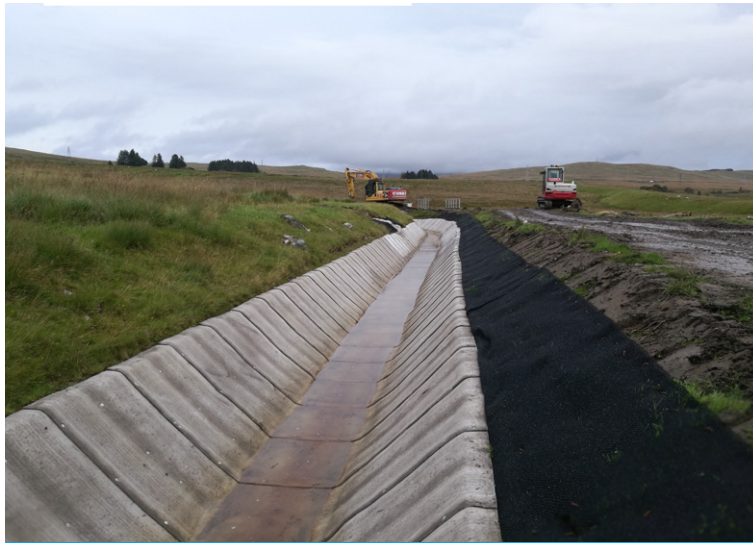
CC layers overlapped in the direction of water flow providing natural weep paths
