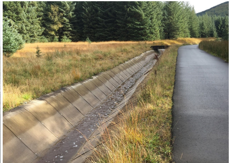
Original Bowburn Flume 4 years after installation requires minimal maintenance
