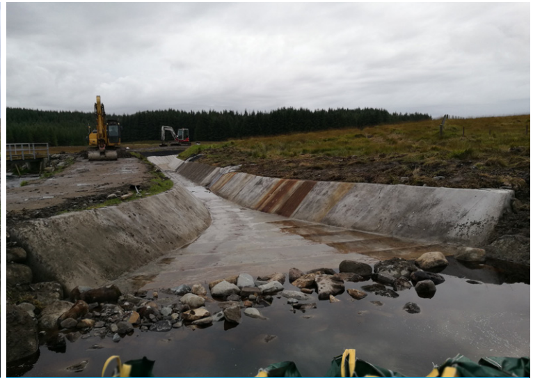
Flume inlet with an anchor trench running across the width of the channel
