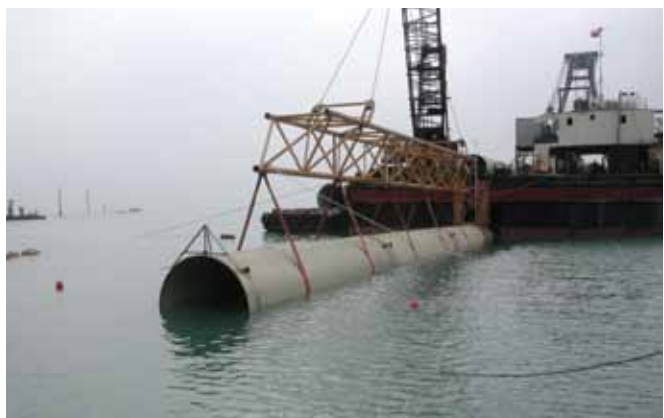
Figures top down: Thrust-bearing pipe installation, non thrust-bearing pipe installation, jacking installation, subaqueous installation
