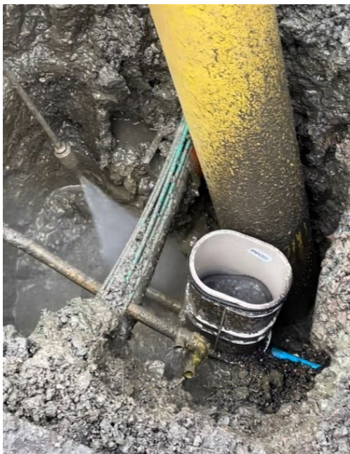
Pressurised water is used to dislodge the ground and loose material is removed up the vacuum hose, the lance has an oscillating nozzle.
