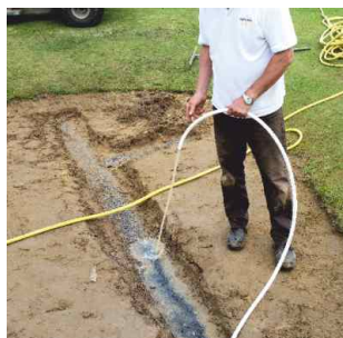
Testing of Enviroflow (1.00 pm)
