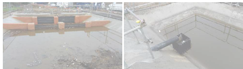
The completed Enviroflow filtration scheme showing all 3 stages of treatment
