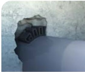
Anchoring the pipe to a concrete wall such as a manhole or tank.
