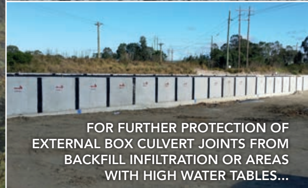
DENSOSTRIP USED TO SEAL BURIED PRECAST CONCRETE TRENCHES DELIVERING SERVICES TO A HISTORIC WATER FOUNTAIN (LEFT)
