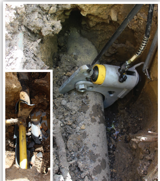
In operation, and on completion of cracking a section of 4" cast iron main
