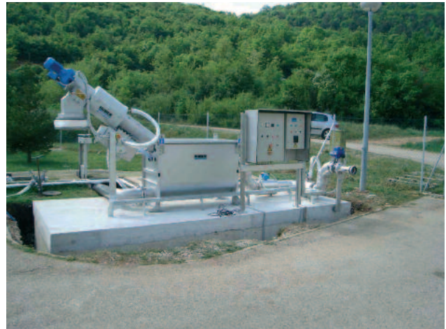
HUBER Sludge Accpetance Plant ROTAMAT® Ro3.1 with HUBER Fine Screen ROTAMAT® Ro1
