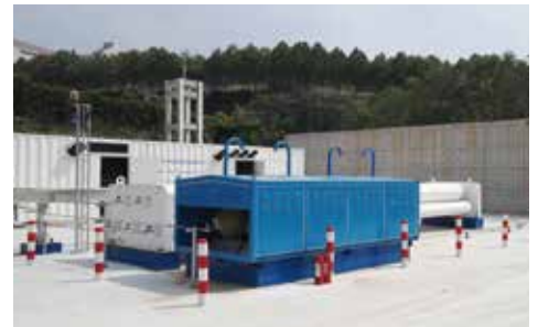
Hydrogen Storage Vessels delivered to the Dalian Tongxin Hydrogen Refueling Station
